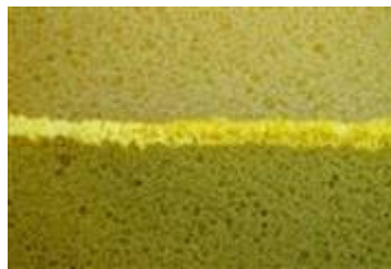
Foam layers glued badly, to thick layer of glue so ventilation becomes a problem.
